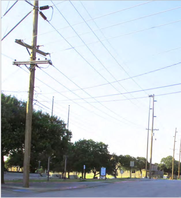
Existing Maple Street electrical transmission poles
